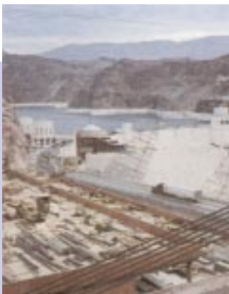
New visitor center rises from a deep V-cut in the canyon wall. Drum-shaped structure is clad with precast panels, some of which follow the profile of rocks and abut.
